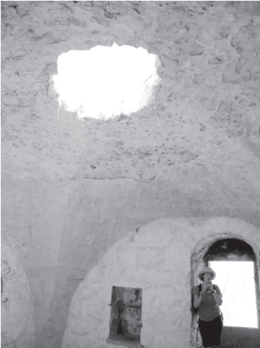
Work day in Lifta: Conducting an alternative survey, 1 June 2012. The holes in the ceilings were made by the Israel Land Administration in the 1960s. Source: Zvika Orr.
